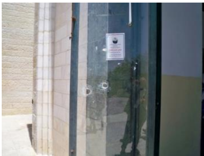
Figure 23: Bullet holes at the entrance of a building, Abu Dis Campus of Al-Quds University, remnants of routine incursions by Israeli police and military (May 2015)
